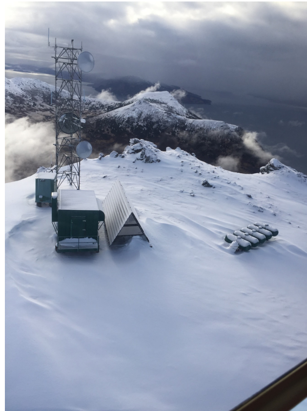
Rescue 21 RFF site in Alaska
