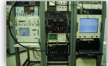
21 m Station Control System
