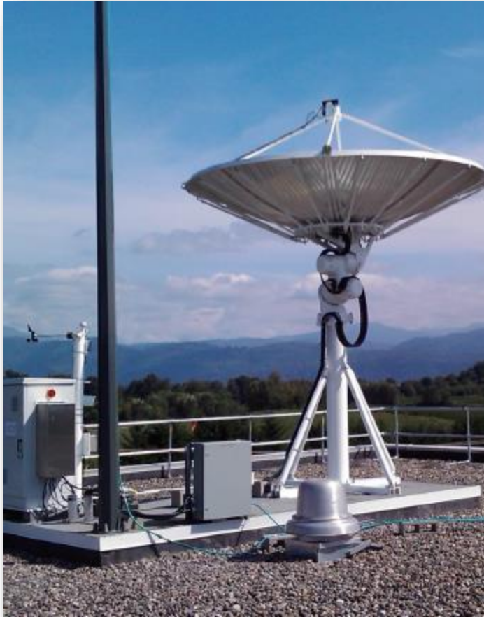
Type 2 Ground Mount on Roof
