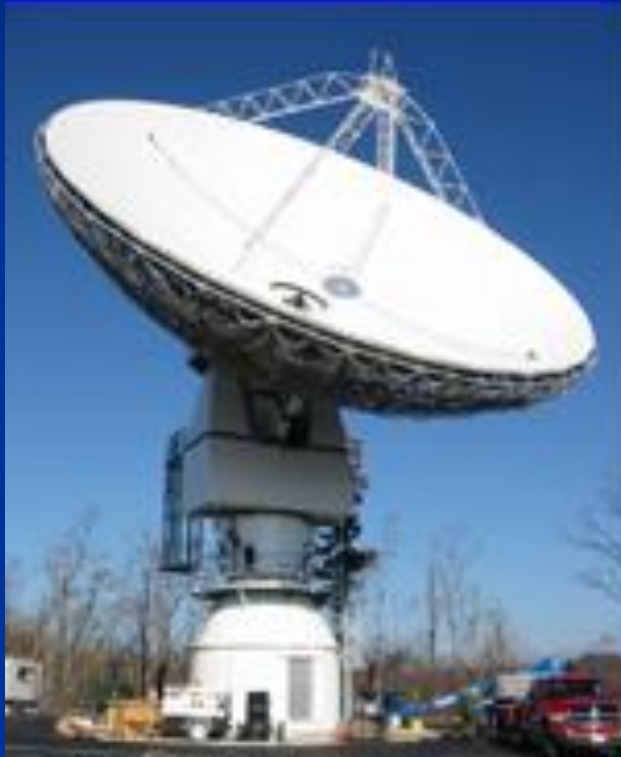
21 Meter Ku band Tracking antenna
