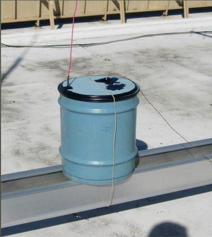
GOES data collection platform container
