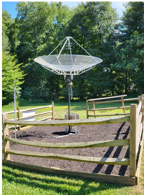
Fig 14: Delaware CubeSat Ground Station
