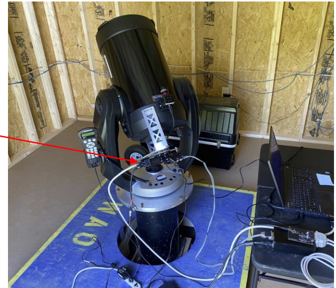
PorTel Optical Ground Station
